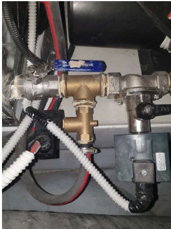
FIG. 5-1. Opening and closing valve of the fuel flow
